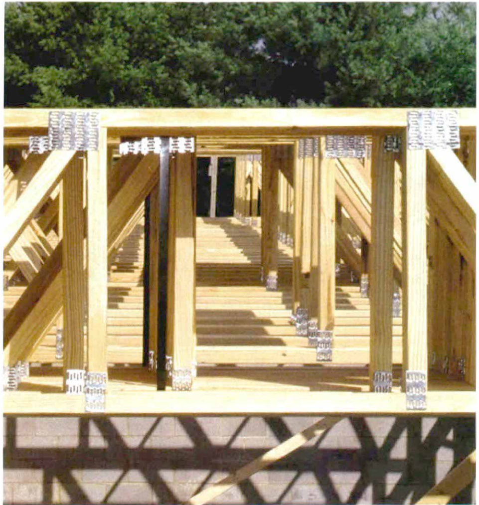
This square chase doesn't align. Several trusses were inadvertently installed backward and had to be reversed so that the square duct chase would align.
