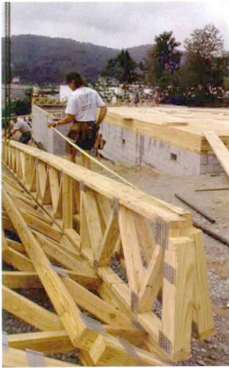
Make sure you get what you ordered. After inspecting each truss for damage, the author measures the trusses to make sure they're built according to the framing plan.
