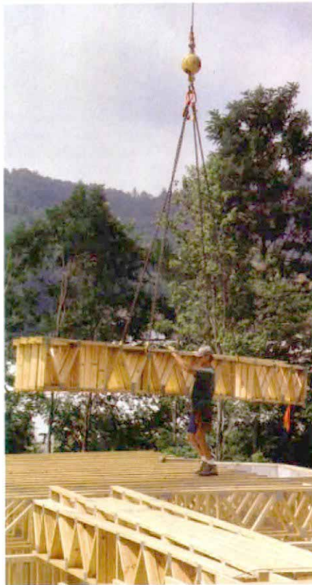
The sling distributes the weight in fourths. With one-quarter of the length of the truss remaining on each end, the crane sling connects to heavy pieces of rebar slipped through the webbing. A worker steadies the trusses and turns the bundle to ensure the trusses all face the right way.
